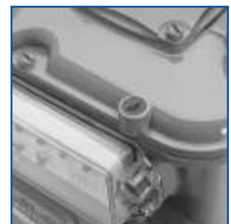
Broken security seal showing evidence of tampering.
